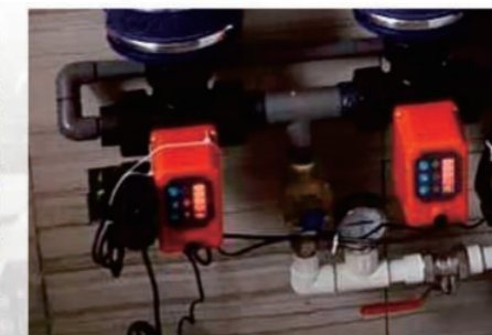
◎反渗透设备 Reverse osmosis equipment
