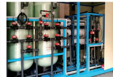
◎超纯水处理系统 Ultrapure water treatment system
